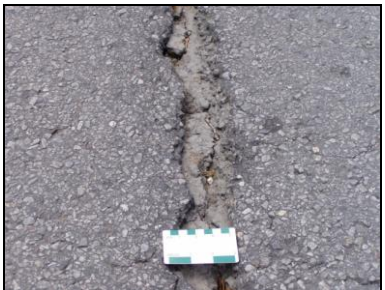
Figure 2.c Severe Longitudinal Cracking
