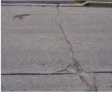
Figure 3a Slight Transverse Cracking
