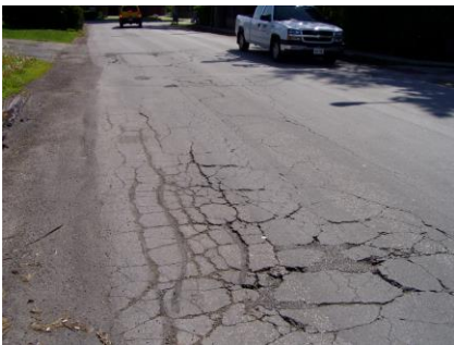
Figure 4c Severe Alligator Cracking
