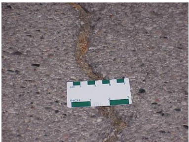
Figure 3b Moderate Transverse Cracking
