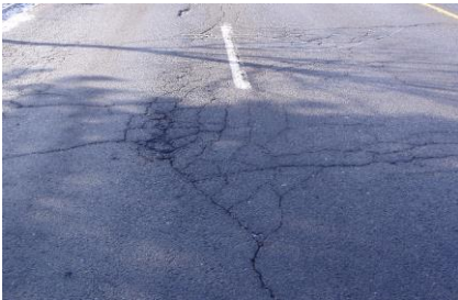
Figure 4b Moderate Alligator Cracking
