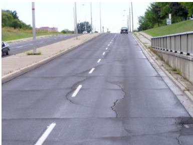
Figure 2.b Moderate Longitudinal Cracking
