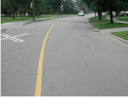
Figure 4a Slight Alligator Cracking
