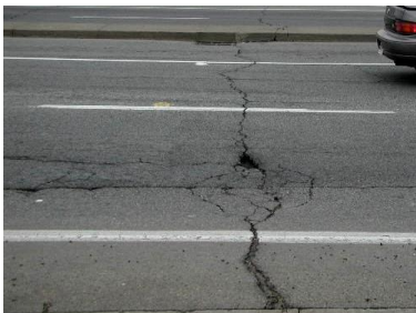
Figure 3c Severe Transverse Cracking
