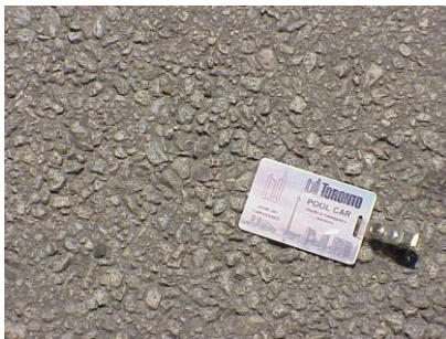
Figure 1a Slight Raveling
