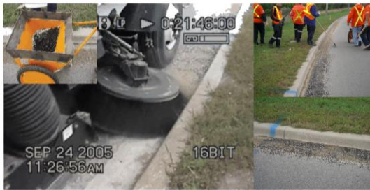
Section E - Heavy Silt Loading Removal (l: 30m X w: 2m)
