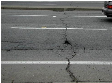
Figure 3c Severe Transverse Cracking
