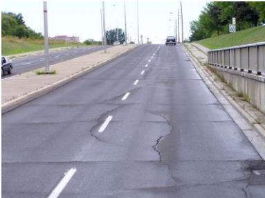
Figure 2.b Moderate Longitudinal Cracking
