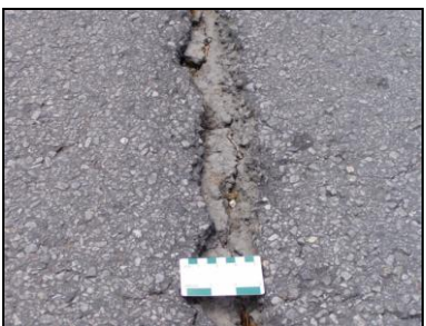
Figure 2.c Severe Longitudinal Cracking
