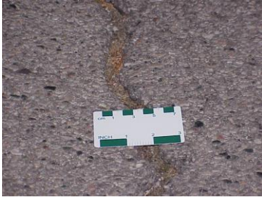
Figure 3b Moderate Transverse Cracking
