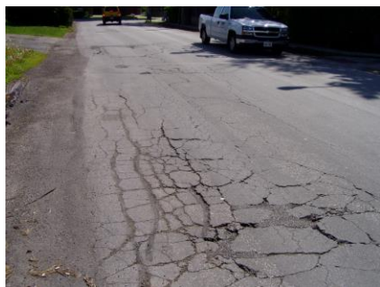
Figure 4c Severe Alligator Cracking
