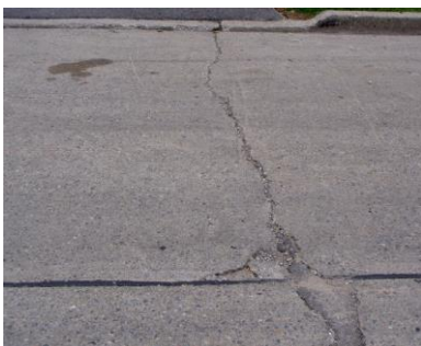
Figure 3a Slight Transverse Cracking
